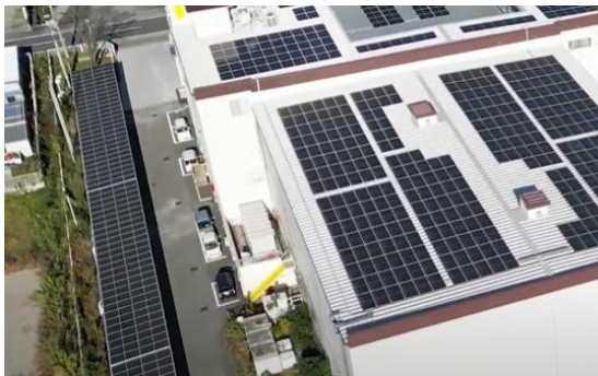
Additional solar panels installed Total 100 million yen
